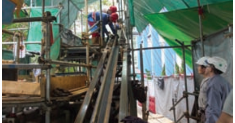
Assembling the STX60 with the straddle packer on the inclined drill rig
